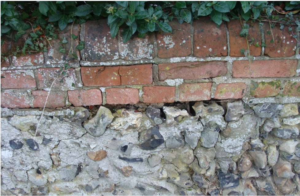
Picture 15 – one of several walls within the curtilages of Listed Buildings at Hadham Ford in need of modest restoration, which if carried out now, will prevent deterioration and additional cost.
