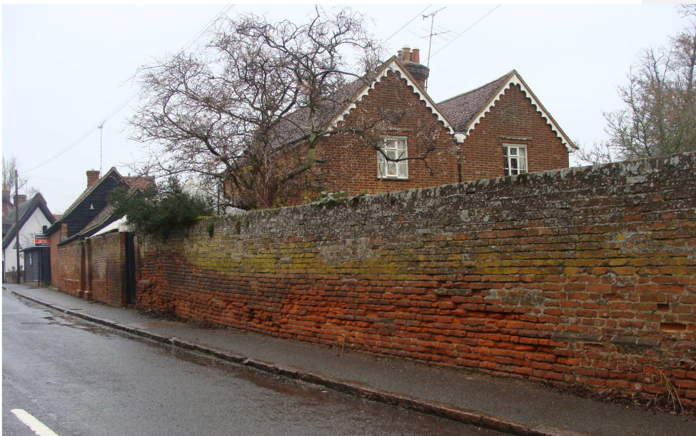
Picture 6 - Quality listed wall considered to be 'At Risk' and in need of repair.
