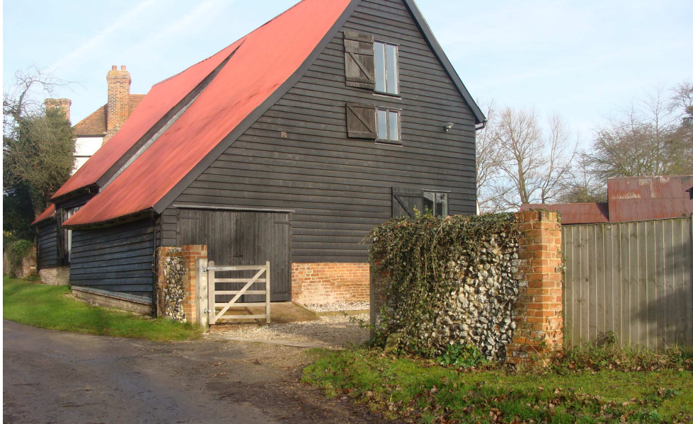
Picture 19 – within the parish there are numbers of roofs with replacement corrugated iron, some of which would originally have been thatched. This one, South Barn at Lower farm is in has been converted to ancillary residential use.
