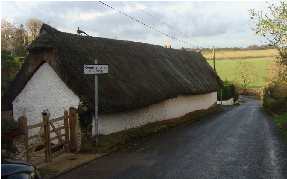
Picture 7 – Thatched building with clay lump walls at Ford Hill. It survives as an obsolete form of building construction of great interest.
